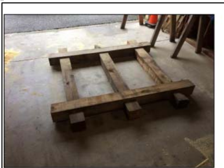
A loon nest platform under construction using 5x5 cedar beams. The platform will be covered with wire mesh and moss prior to deployment.
