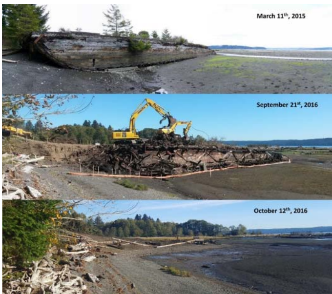
Dosewallips estuary restoration site before, during, and after the work of removing the barge.
