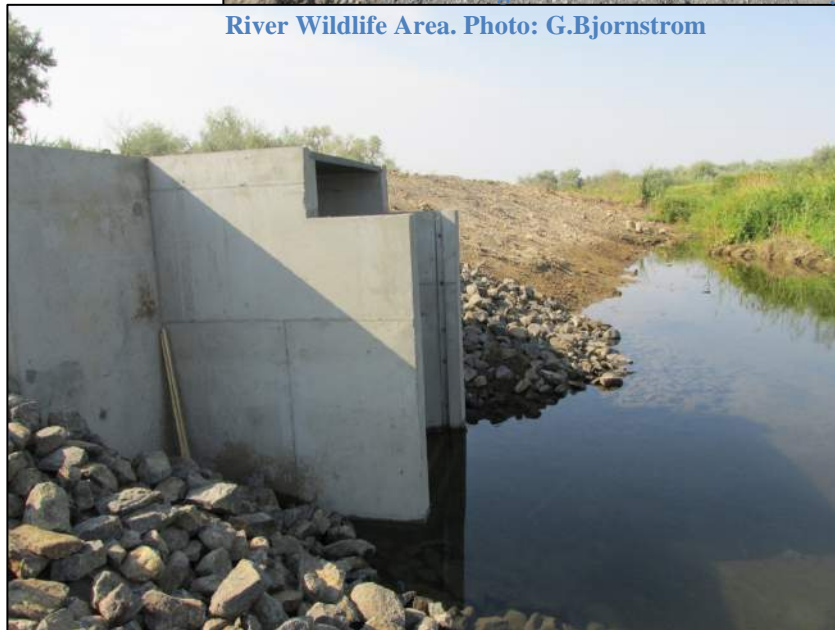
New water control structure at the West Pigeon Pond - Mesa Lake/Sunnyside Snake River Wildlife Area. Photo: G. Bjornstrom
